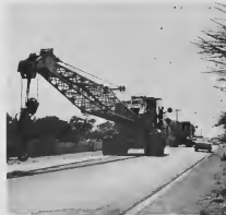
MOTORISTS HEADING toward San Nicolas were greeted with this strange sight, above, as the cranes rolled to Oranjestad. The tank, below, was slipped off the barge.
